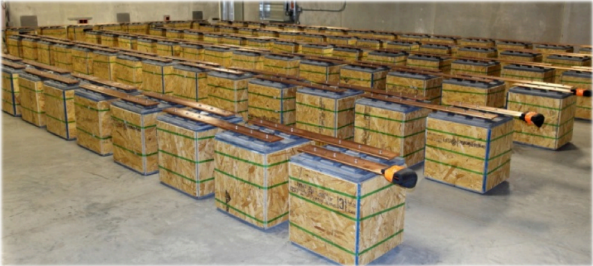
Large Grid Storage Device (approx. 1MW)
