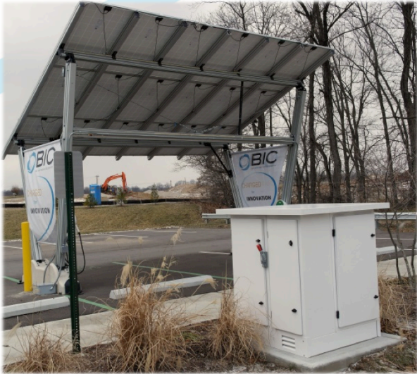
Integrated Power System (IPS) Supporting Solar and Wind Data Collection and Remote Management
